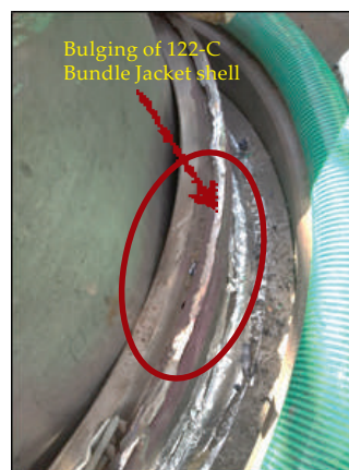
Figure 5. Bulging of 122-C bundle jacket shell
