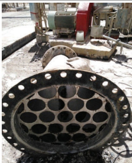
Figure 3. Installation of suction strainer to high flow slurry pump associated with 3 rd reactor
