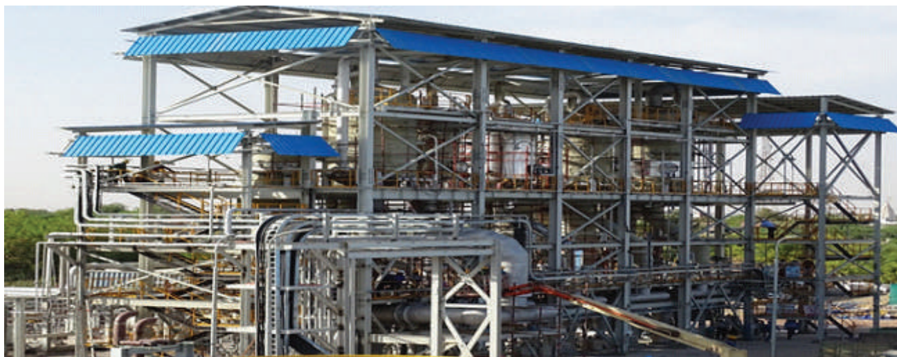
Figure 8. Photograph of ZLD plant
