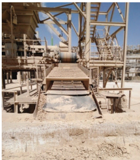
Figure 1. An image of vibrating screen on-line in rock feeding system
