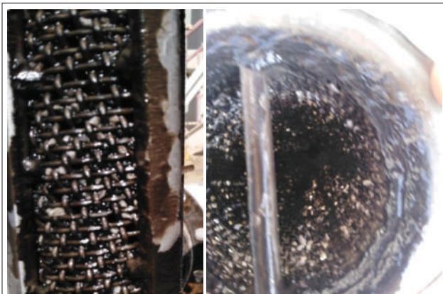
Figure 4. Black sticky material was observed in the circulation acid system. Strainers were accumulated with this black material.
